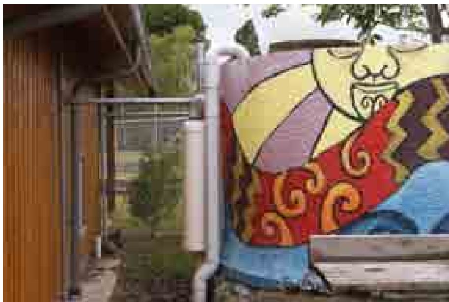
The water tank for garden irrigation
